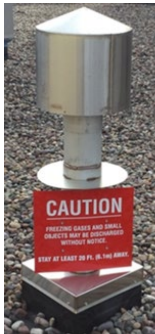
FIGURE 5. Example of a cryogen vent with signage.
