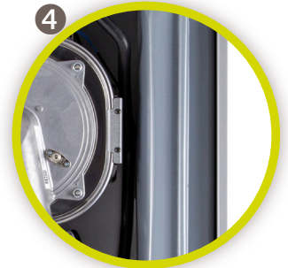
Heating expansion vessel
