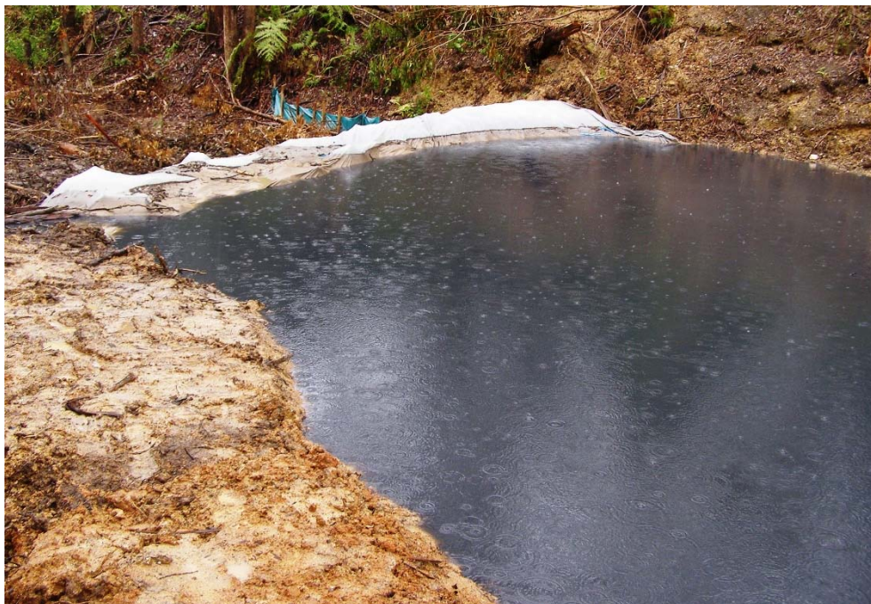
Plate 4: Tannin impact in stormwater at the discharge point from a road construction site. The discharge of impacted water may be obvious to community and other stakeholders.
