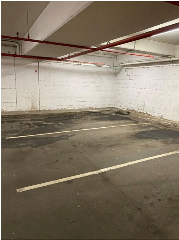
St Marys Plaza Underground Carpark oil staining
