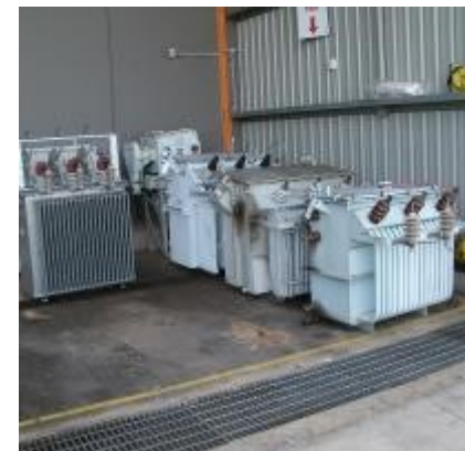
Old distribution transformers within bunded area
