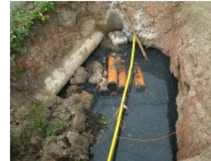
Contaminated water requires removal by an EPA licensed liquid waste contractor
