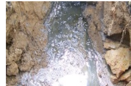
The presence of an oily sheen is a sign of potential contamination
