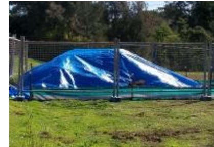
Stockpiles of acid sulfate soil should be covered with plastic
