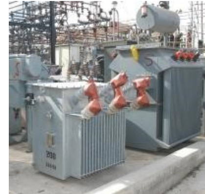
New transformer storage
