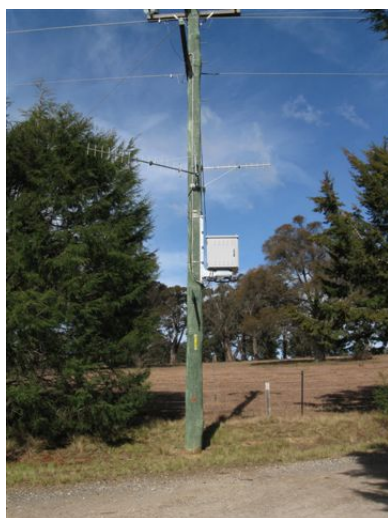
a) Endeavour Energy communication repeater enclosure
