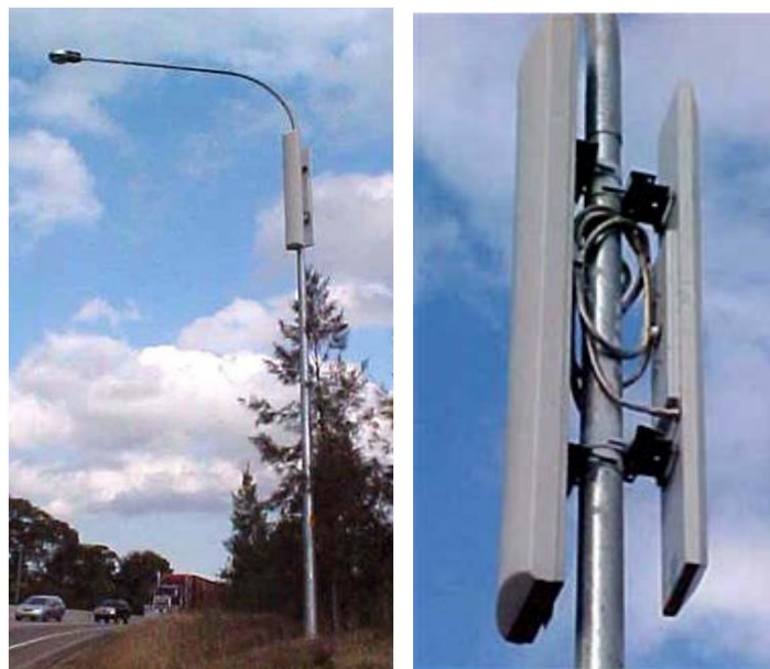
Figure 11 : Installations of antenna for mobile phone cells
