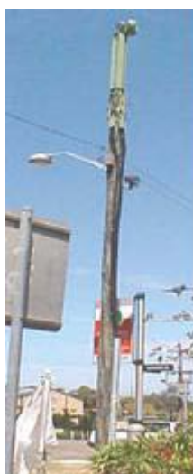
b) Mobile phone cell attachment with communication cable along the pole
