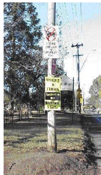
Figure 6: Unacceptable sign clutter, creating pole climbing hazards and obstruction to pole inspections
