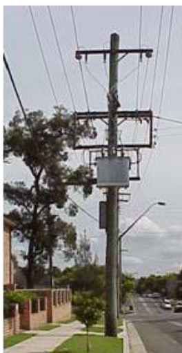
b) A pole with a substation
