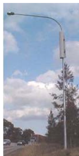
c) Mobile phone cell attachment on steel street light pole
