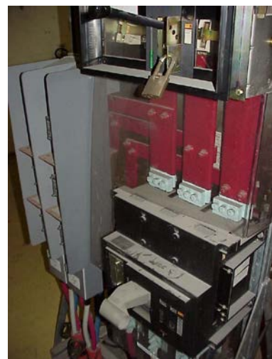
Figure 6 - Cover on busbar to CB connections
