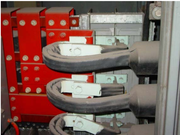
Figure 2 - Cover over connections at busbar + fuse strip
