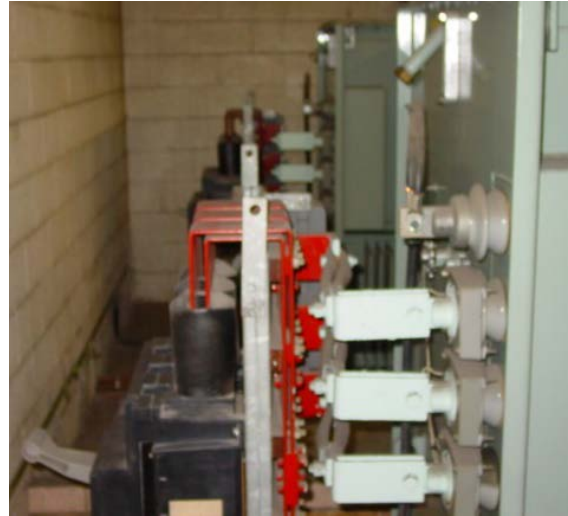
Figure 3 - Cover on bushing to LV busbar connection 1
