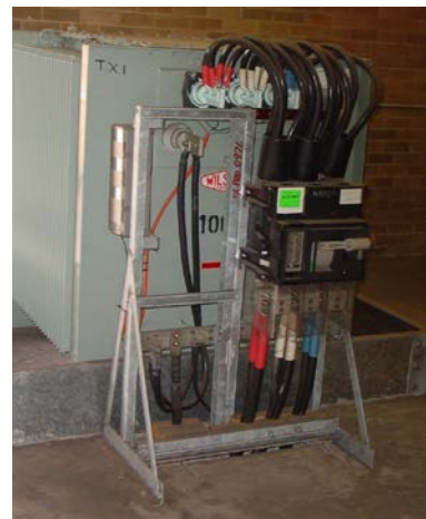
Figure 5 - Cover on top connected LV bushings
