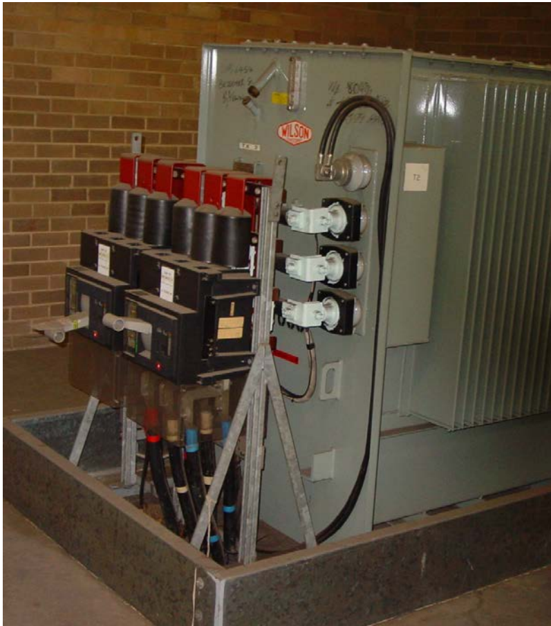
Figure 4 - Cover on bushing to LV busbar connection 2
