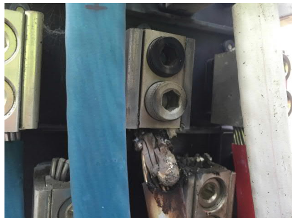
Figure 2: The failed “B” phase connection with the bottom screw not sufficiently tightened.
