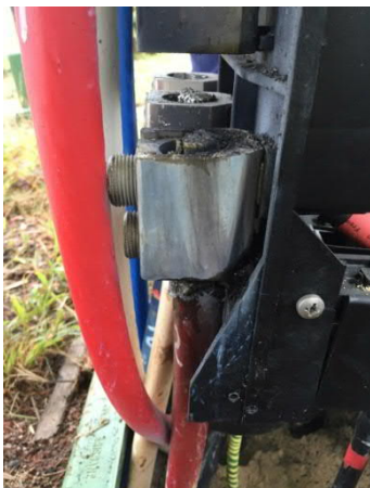
Figure 1: The failed “A” phase connection with top screw not sufficiently
