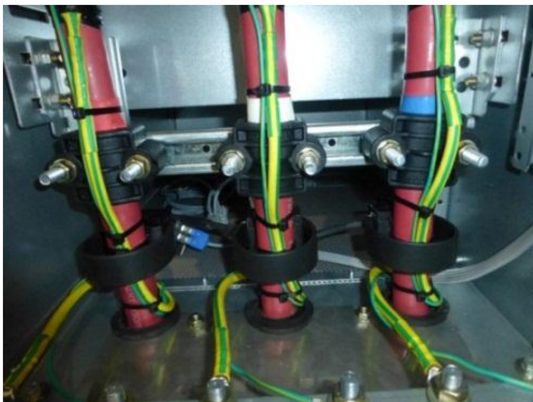
Figure 6-All CTs are to be level and with the cable passing through the centre of the CT core
