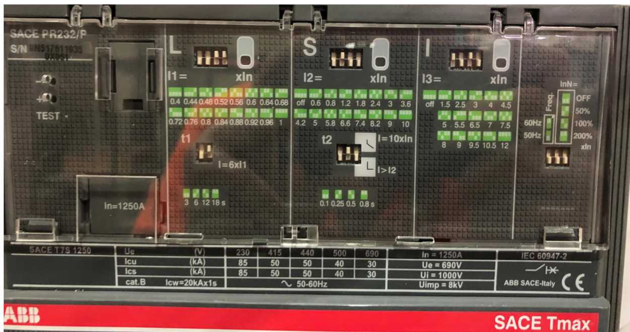
ABB PR232 T7 1250 for 315kVA Transformer
