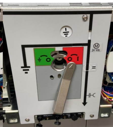
Figure 3. Selector switch allowed to travel clockwise and lock in. Defective mechanism.
