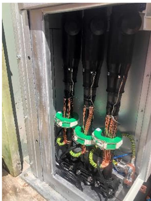
Correctly installed CTs in an ABB Safelink
