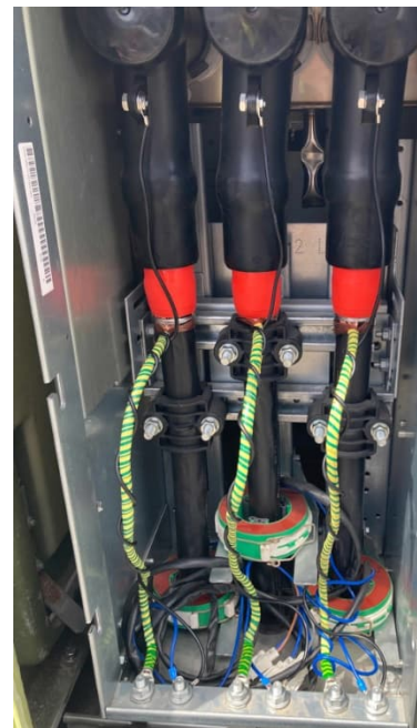
Incorrectly installed CTs in Siemens 8DJH
