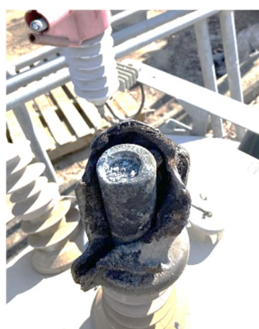
Fig. 1 OSM 200 series failure
