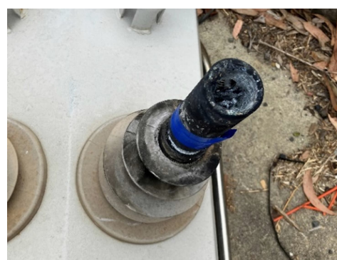
Fig. 2 OSM 300 series failure
