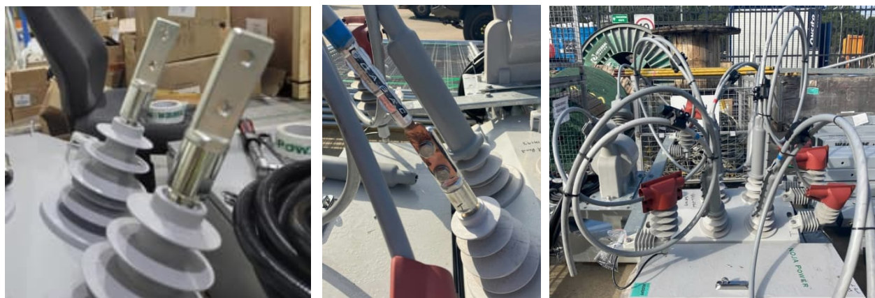
Fig. 3 Photos of palm terminal and the bi metal lug
