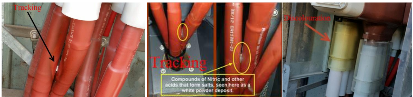
Figure 1: Physical signs of Tracking and Discolouration
