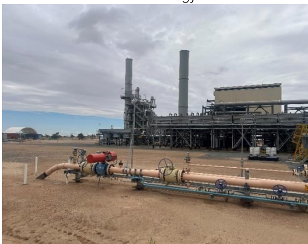
Picture 2: CO 2 Pipeline
