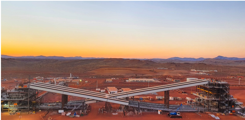
Ore processing facility
