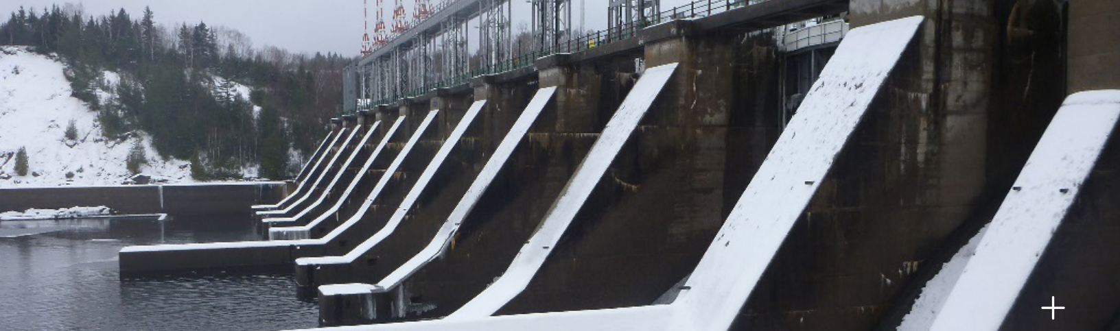
Grand Falls, Beechwood, and Tobique Developments Flood Study and Dam Safety Review
