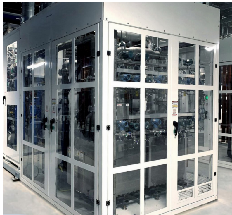
Electrolyzer installation inside the Air Liquide Bécancour Hydrogen Complex
