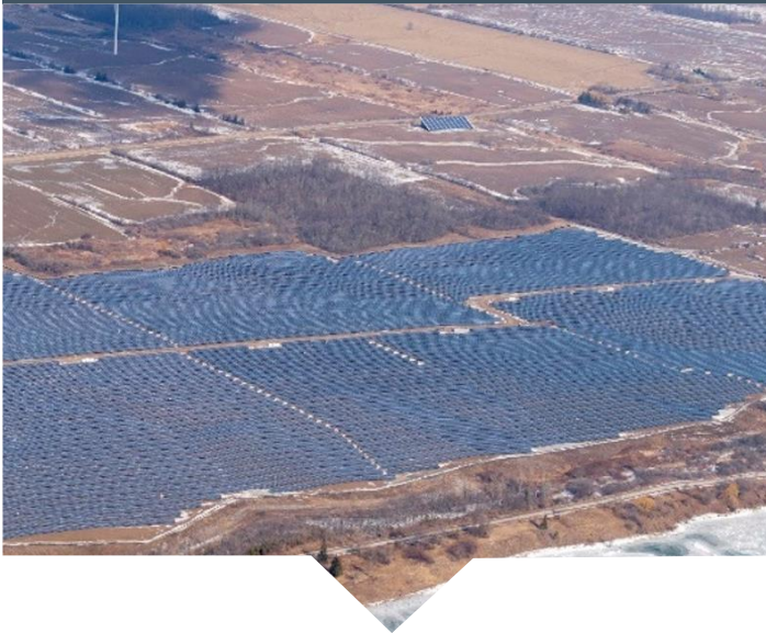
Nanticoke 44MW Solar PV Power Plant
