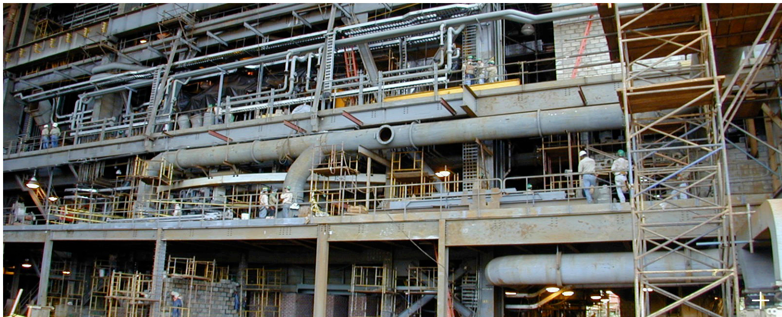
The Cerro Matoso ferronickel plant doubled its capacity with the addition of a second rotary kiln electric furnace line.
