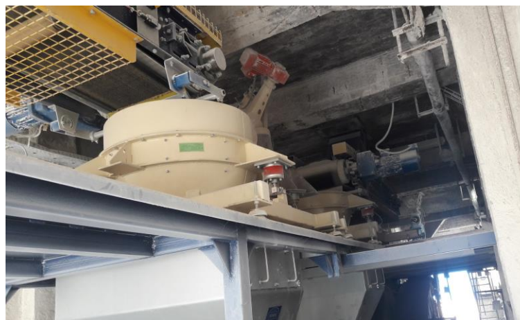
New dosing system (lower raw materials consumption).
