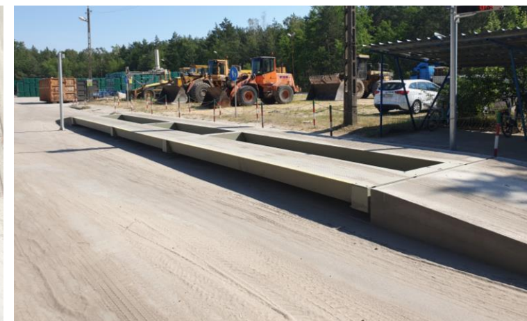
New truck scale (better control of raw materials delivered).
