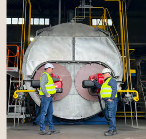
Przemysław Sztaboroski and Marian Misztela inspect the steam boiler converted from using coal to now using natural gas through the yellow pipes.
