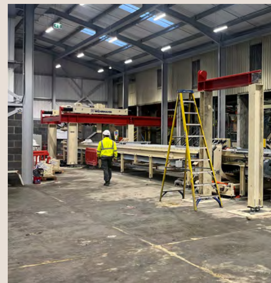
Picture of the expansion works at the Borough Green plant in the UK which began end of 2023.
