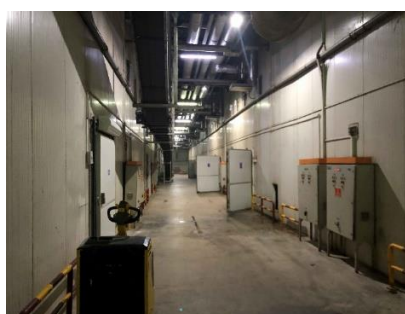
Cold rooms, CA storage and ripening
