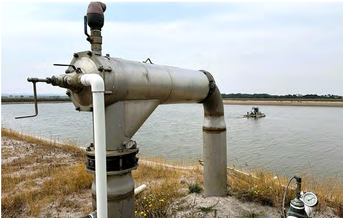
Figure 14. Surface water drawn from rivers is stored in farm ponds for sediment settlement and passed through a coarse filtration system.
