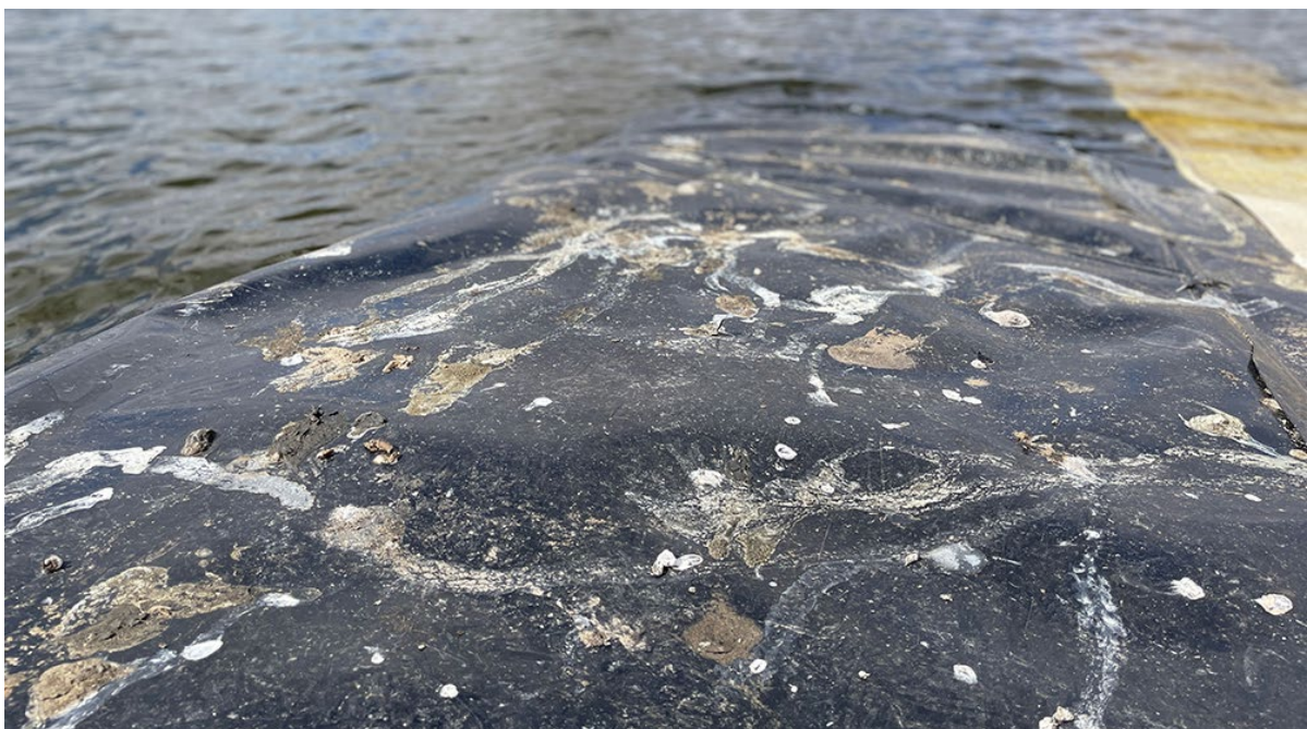
Figure 53. Waterbird activity around an irrigation dam, showing faecal contamination on the dam liner, which is a potential source of biological hazards.
