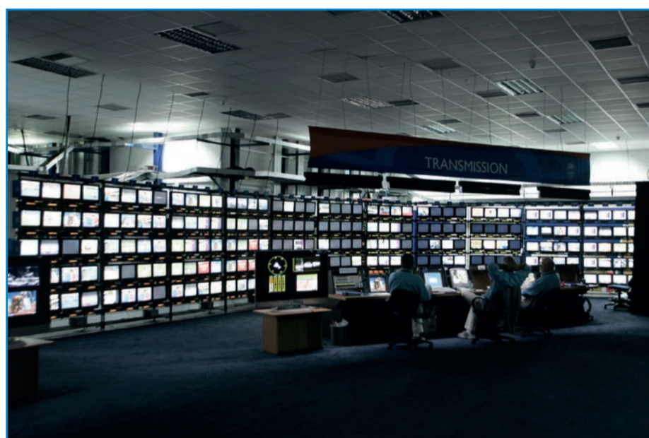
Control room in the International Broadcast Centre.
