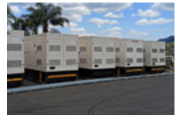
LOAD SHARING GENERATORS
