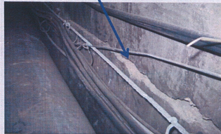
Crack in South Wall
