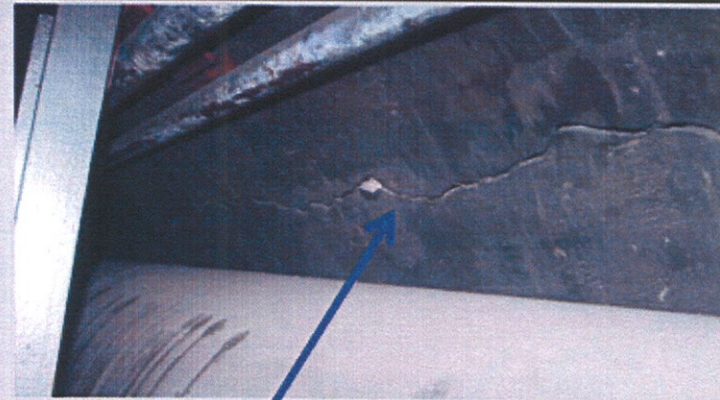
Crack in North wall
