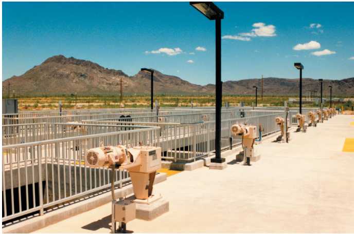
HT agitators working to treat waste and suspend solids at an Arizona treatment facility
