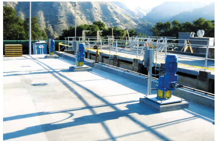
Colorado water processing plant utilizing Model 20 GT agitators
