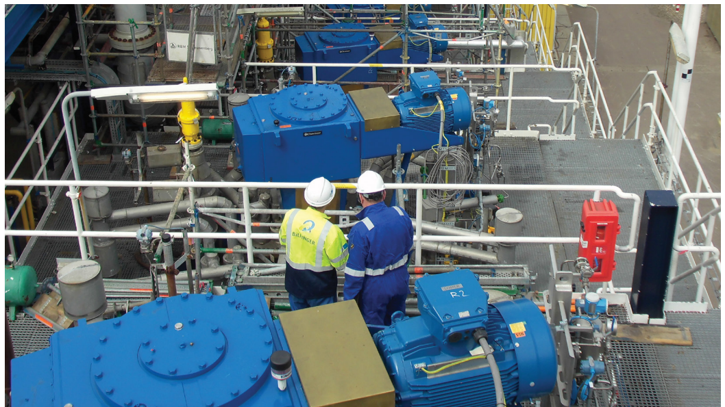
Field service technicians are readily available to help maintain your equipment as shown in this large chemical plant in the UK
