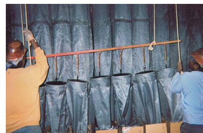
Service personnel changing out bags in a reverse air collector.
