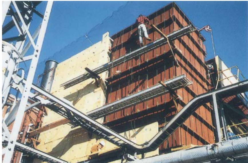
A MikroPul service team stripped this baghouse to its frame, then rebuilt it to new-equipment specifications in half the time and at half the cost of a new unit.
