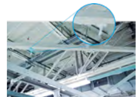
Dust Deposits in Ceiling
