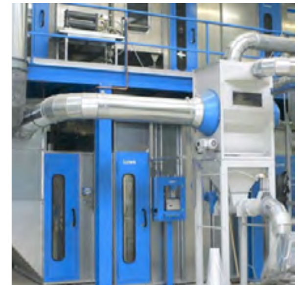
TexPac - Centralized Air Handling System
