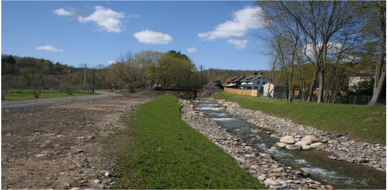
Figure 23. Post construction – View of upstream portion of Steele Creek restoration showing stream channel with in-stream features, floodplain restoration and partial removal of East River Drive. Flood buyouts also occurred to the left, just outside the picture.
