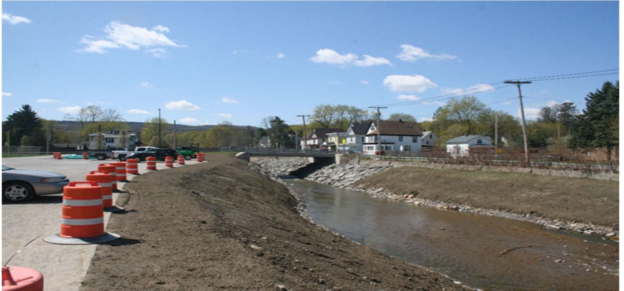
Figure 22. During construction – view looking upstream towards Fredrick’s Street bridge on Steele Creek within the Village of Iliion..
