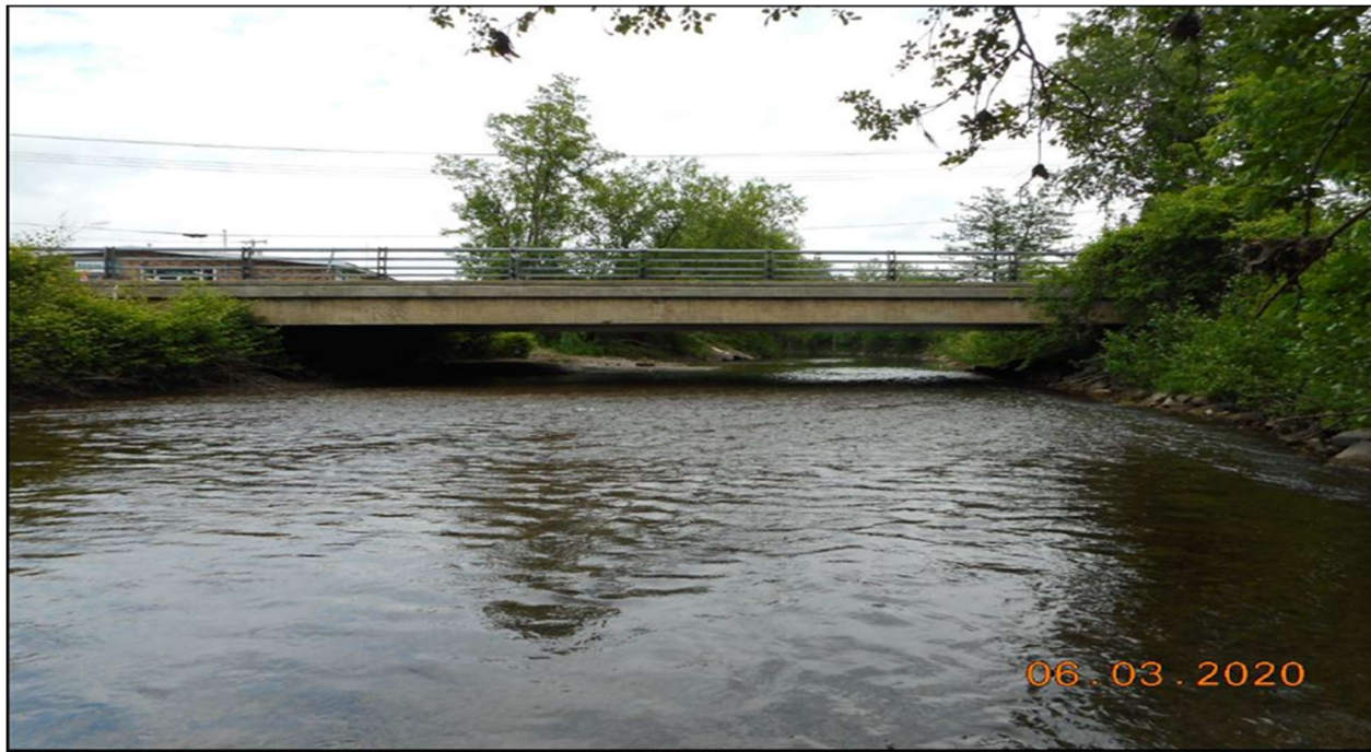
Figure 11. Ground level view of Main Street bridge that will be replaced and upsized by NYSDOT.
