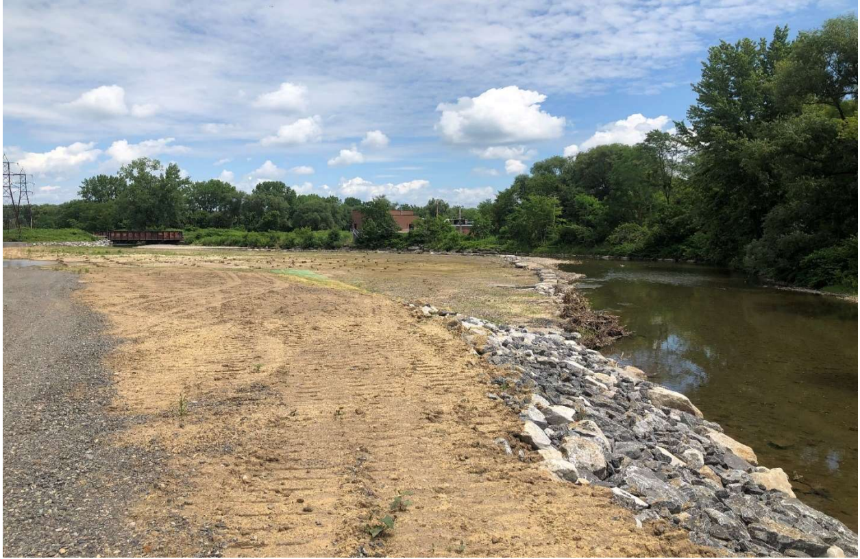
Figure 6. Ground level view of Project 2 floodplain restoration just south of CSX railroad. CSX bridge is in the background.
