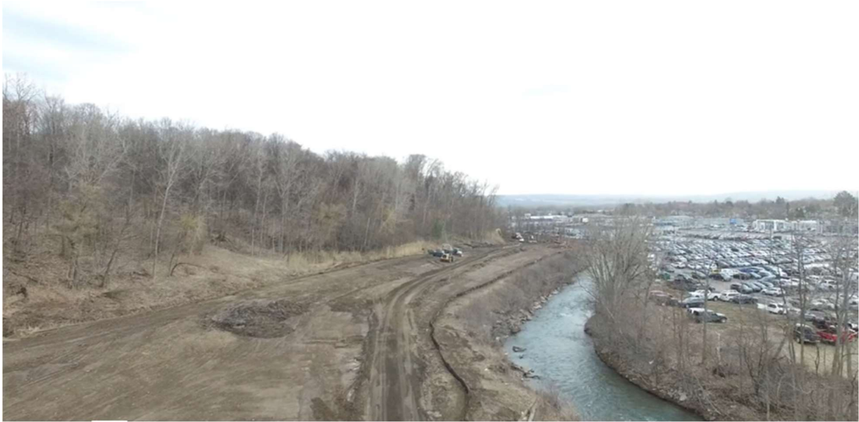
Figure 2. Aerial view of Project 1 underway in Dunham Manor Park, Town of Whitestown.
