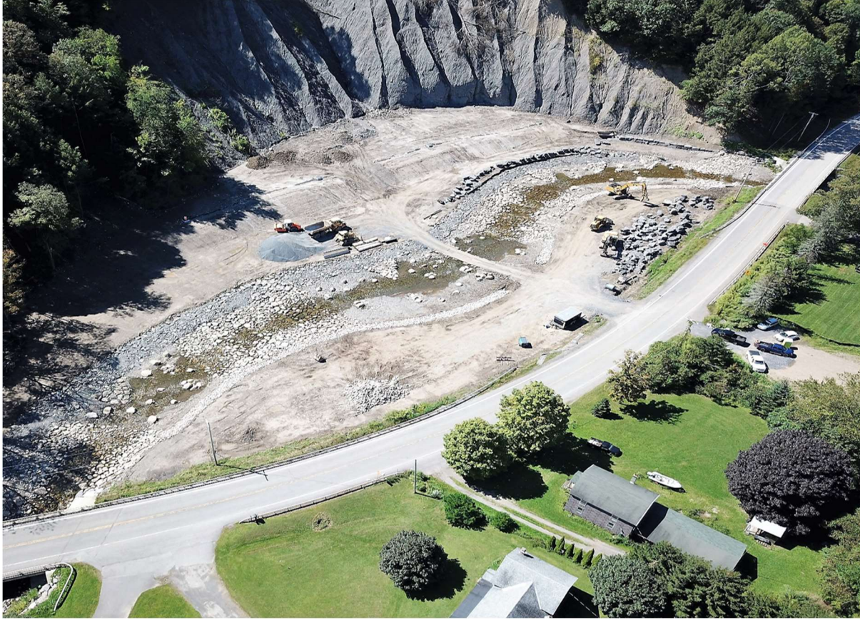
Figure 31. Aerial view of ongoing slope stabilization and floodplain restoration project on Fulmer Creek.
