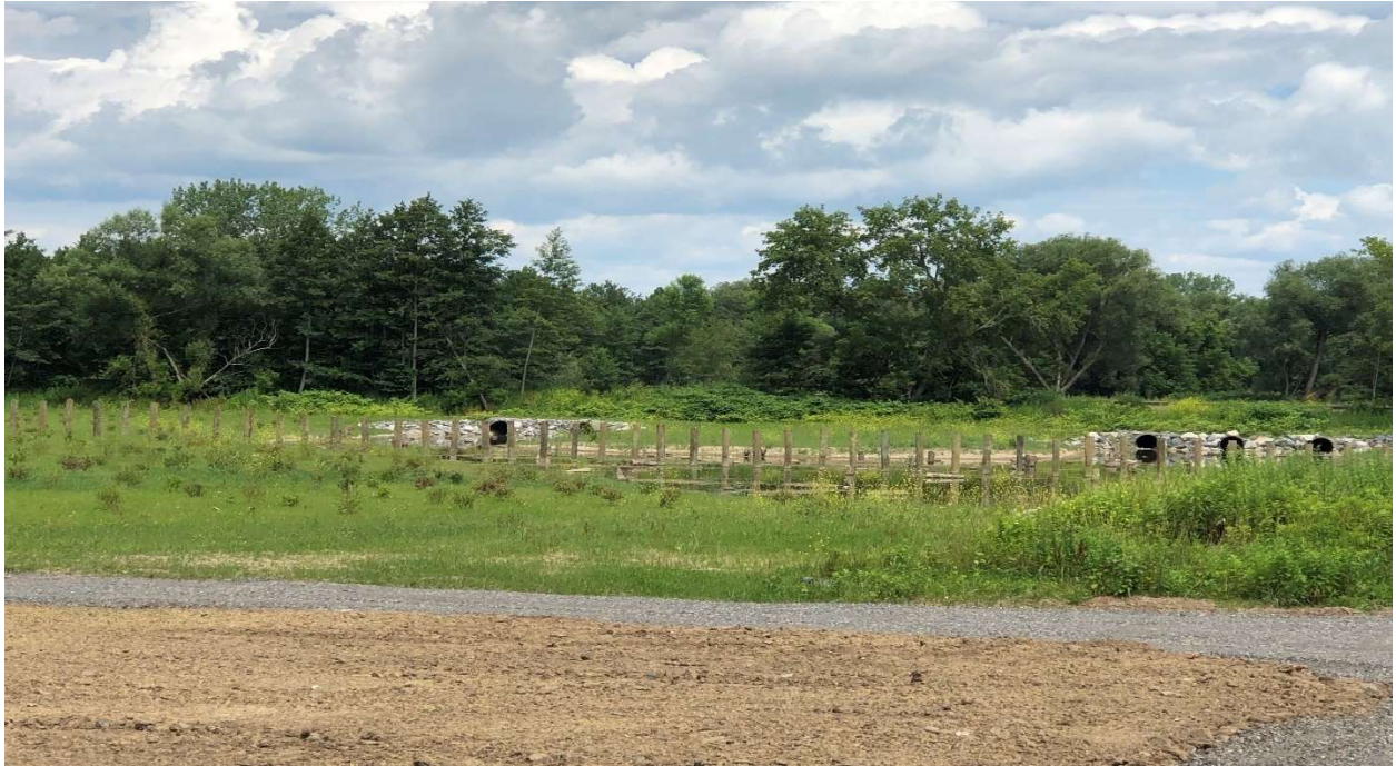
Figure 7. Ground level view of Project 2 floodplain restoration and the installation of five 48-inch culverts in CSX railroad bed.
