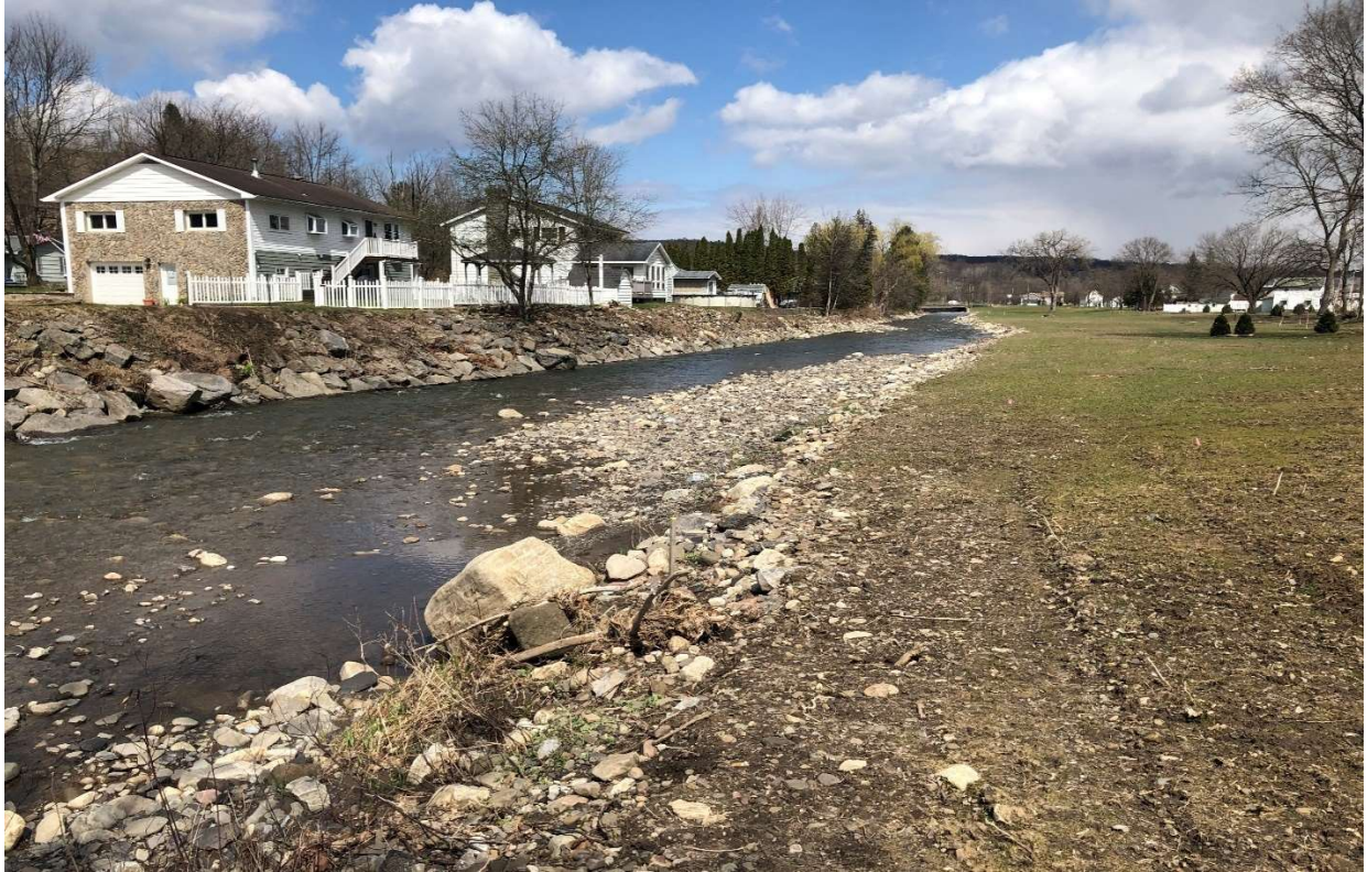
Figure 34. Photo of completed Fulmer Creek floodplain restoration project within Village of Mohawk.
