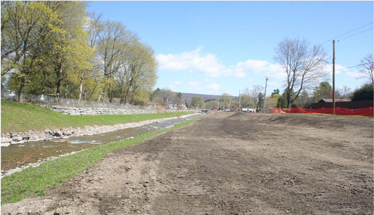
Figure 21. During construction – view looking downstream showing stream channel and floodplain restoration on Steele Creek, Village of Iliion.
