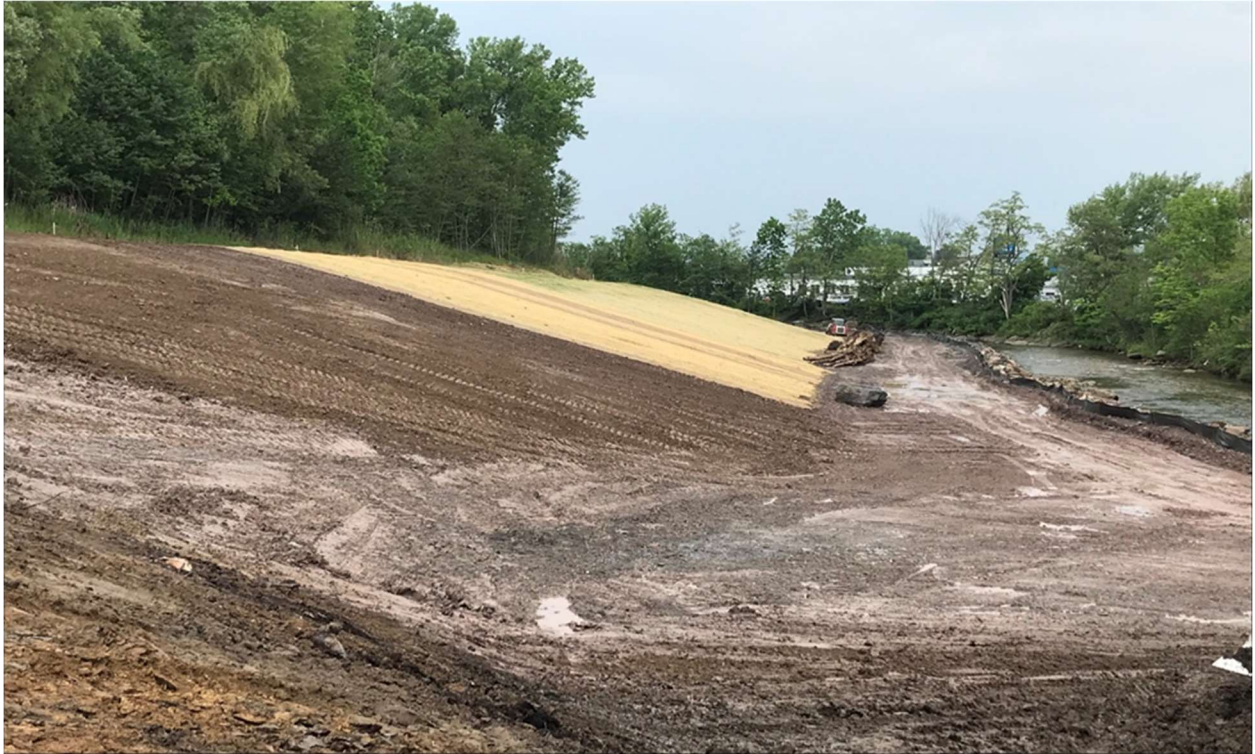
Figure 4. Ongoing construction of Project 1 underway in Dunham Manor Park, Town of Whitestown.
