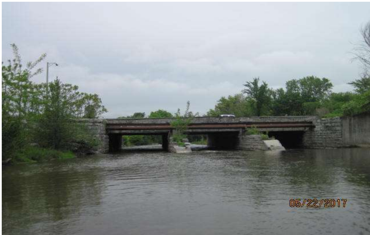
Figure 13. Ground-level view of State Route 69 or Oriskany Boulevard bridge the will be replaced by NYSDOT. This bridge is a chronic source of debris/ice jams due to the remnants of the old Erie Canal Aqueduct adjoining the bridge piers. The old Erie Canal Aqueduct structure will be removed as part of the new bridge replacement to alleviate future debris/ice jams.
