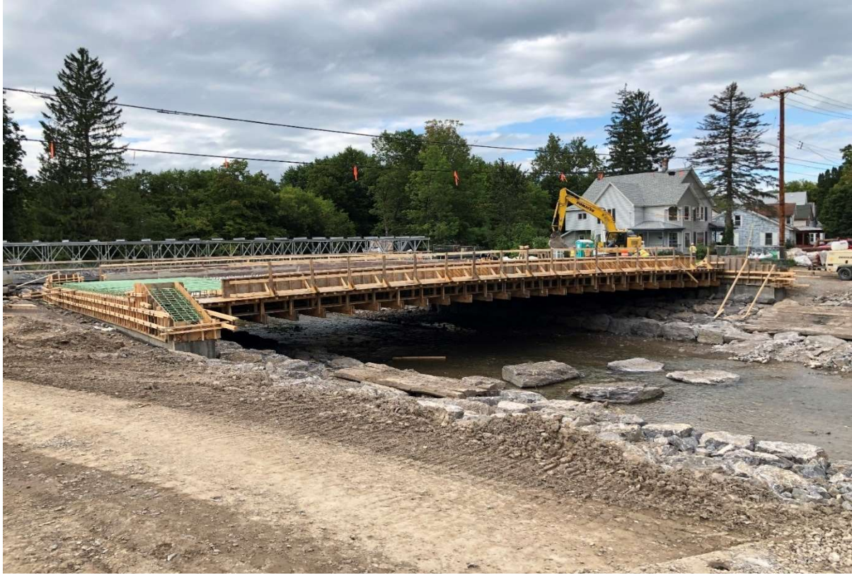
Figure 26 – Photo of new State Route 51 (Otsego Street) bridge being replaced by NYSDOT. Several homes surrounding the bridge were acquired by the Village giving NYSDOT sufficient area to install a significantly larger structure.
