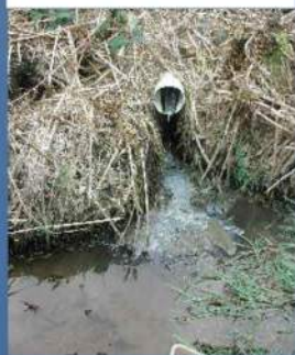
Illicit Sewer Discharges
