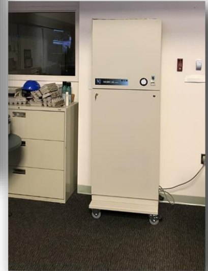
Installed Portable & Permanent Air Filters
