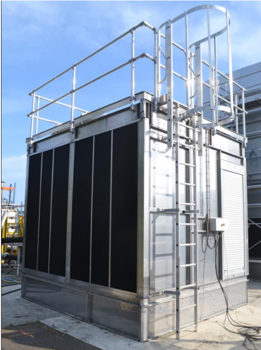
Open cooling tower
