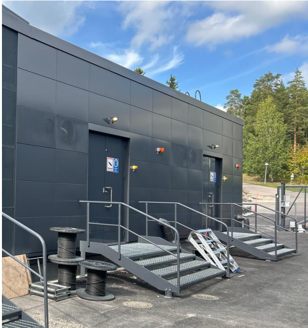
Heat pump modules
