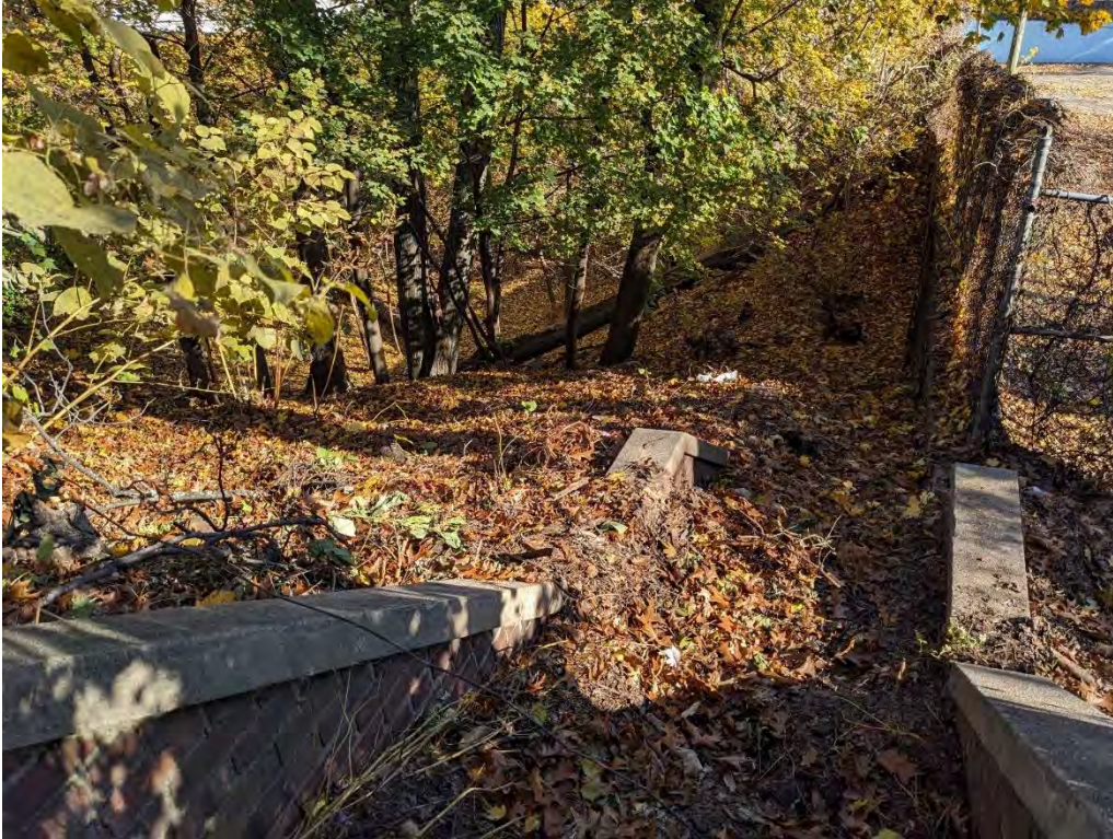
Photograph 15. The steeply sloped area at the northeast corner of the campus. View looking northeast.
