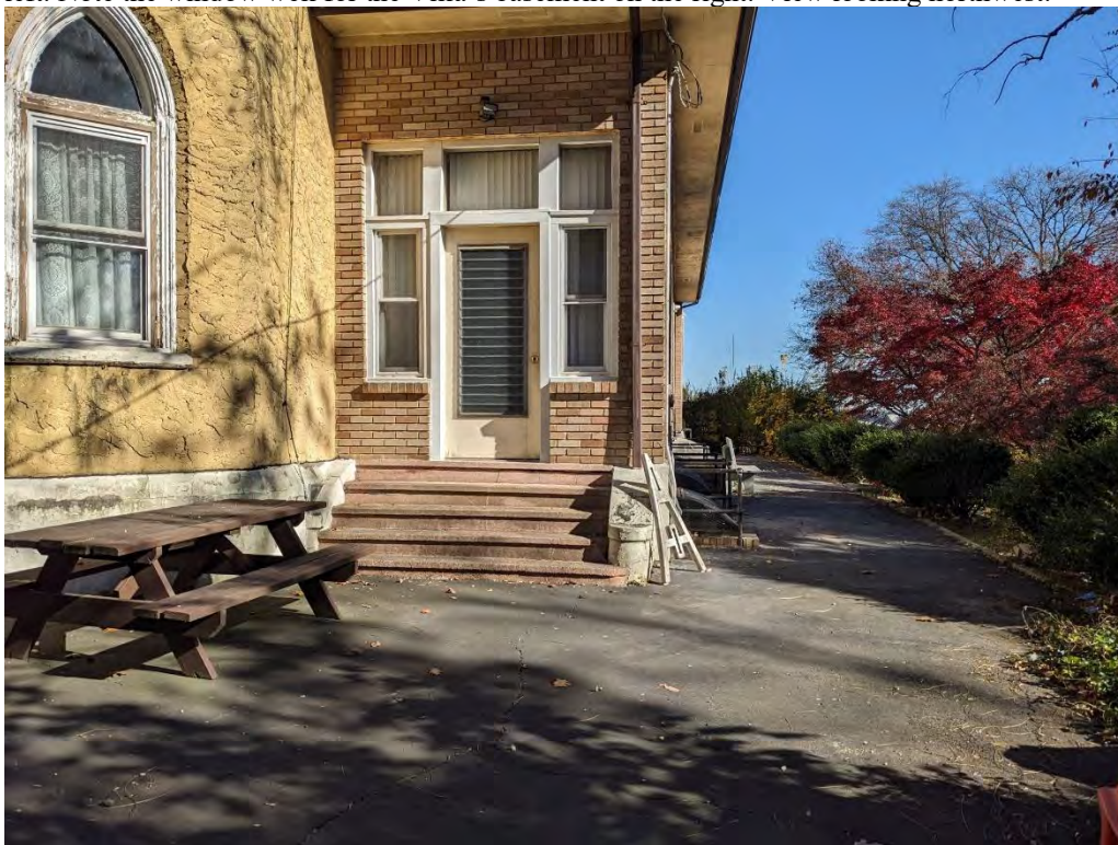
Photograph 4. The rear of the former Villa, showing the former location of the wraparound porch that has been enclosed as an addition with a full basement. Window wells to the basement are located along the edges. View looking northeast.
