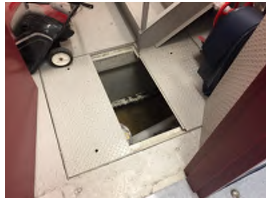
Figure 2: Backwater Valve located in the Utility Room.
