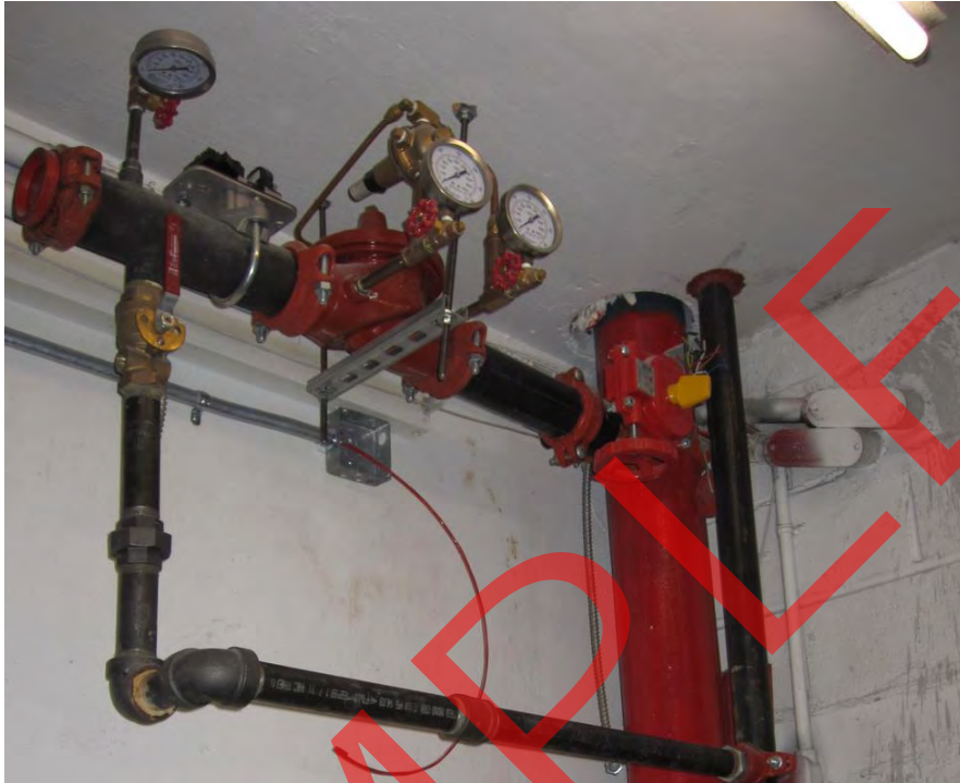
Photo PF-2: 4" sprinkler floor control valve station
