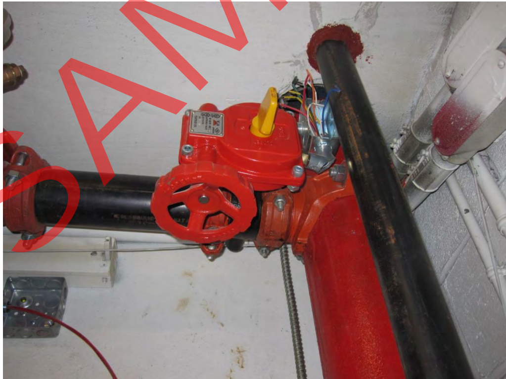
Photo PF-3: Incomplete installations of tamper switch wiring and alarm wiring
