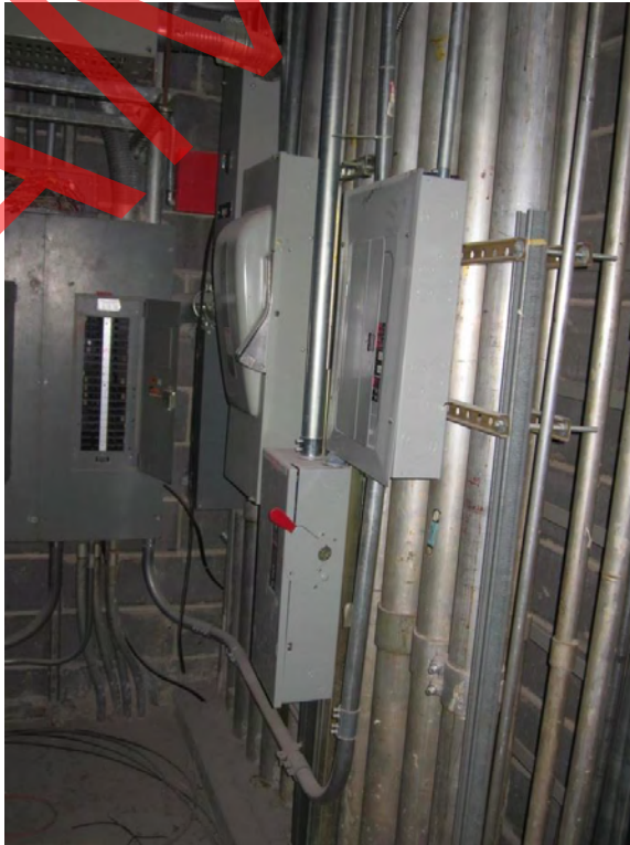
Photo E-2: Electrical panels and a transformer in electrical room
