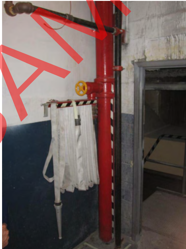
Photo PF-1: 6" combined standpipe/sprinkler riser with 2.5" fire department valve and 1.5" hose
