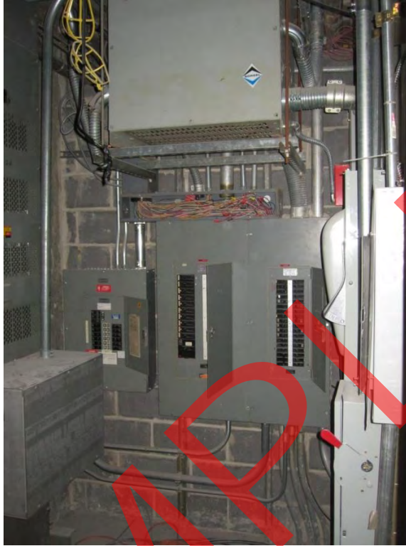
Photo E-1: Electrical panels and a transformer in electrical room
