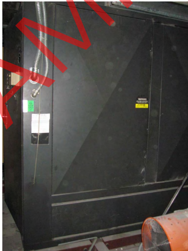
Photo M-8: Indoor air handling unit in fan room
