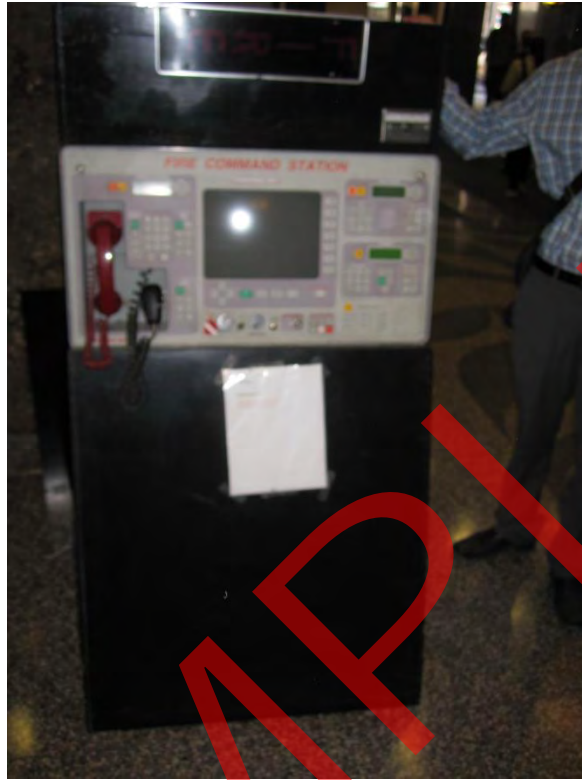
Photo FA-2: Central fire alarm command station in 1 st floor lobby
