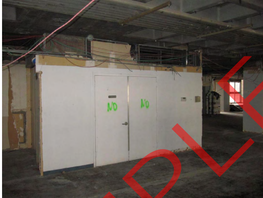
Photo M-7: Existing 2 nd floor interior fan room
