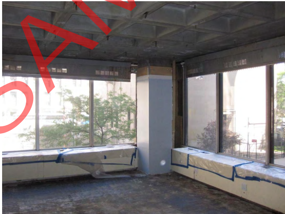
Photo M-2: Perimeter induction unit in metal cabinetry below the windows
