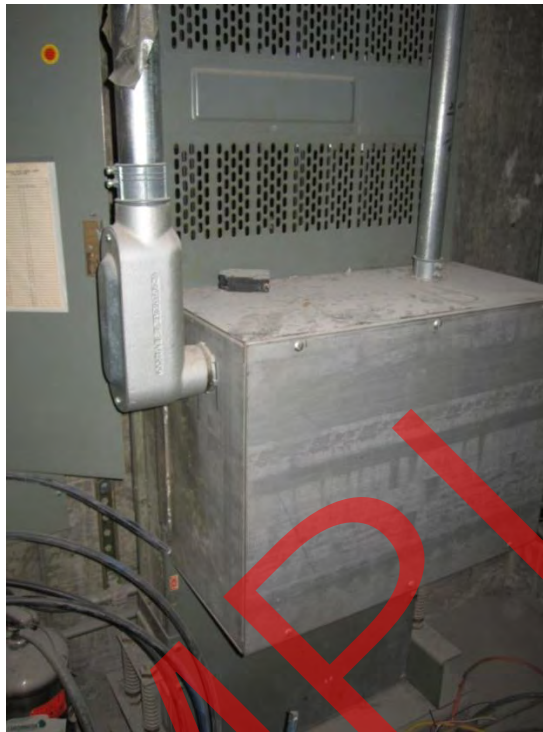
Photo E-3: Buss duct rises vertically through the electrical room
