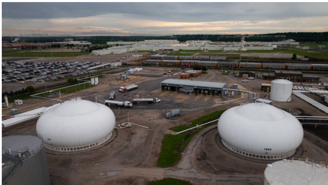
Figure 3: Refined products storage tanks and ancillary infrastructure at our Kansas City, Missouri, facility are critical to providing uninterrupted fuel supply across our contiguous systems for the transportation and agricultural sectors, among others.
