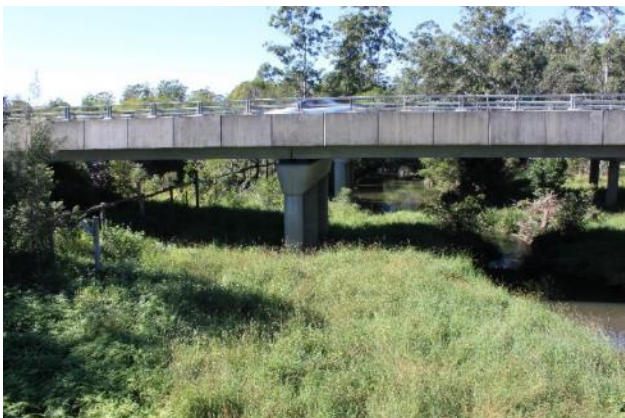
E) Extended bridge underpass across floodplain and river along Pacific Highway, Northern NSW.
