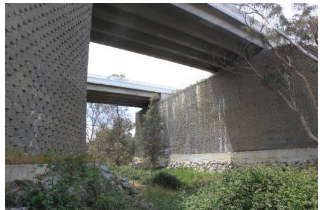
F) Combined drainage and fauna underpass at Forest Creek, Calder Freeway, Vic.
