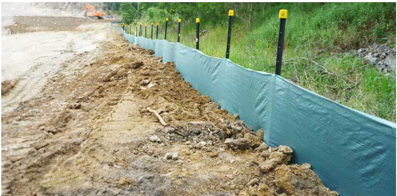
Photo 10.2 Example of construction phase silt/sediment fence (source: AussieEnvironmental.com.au)
