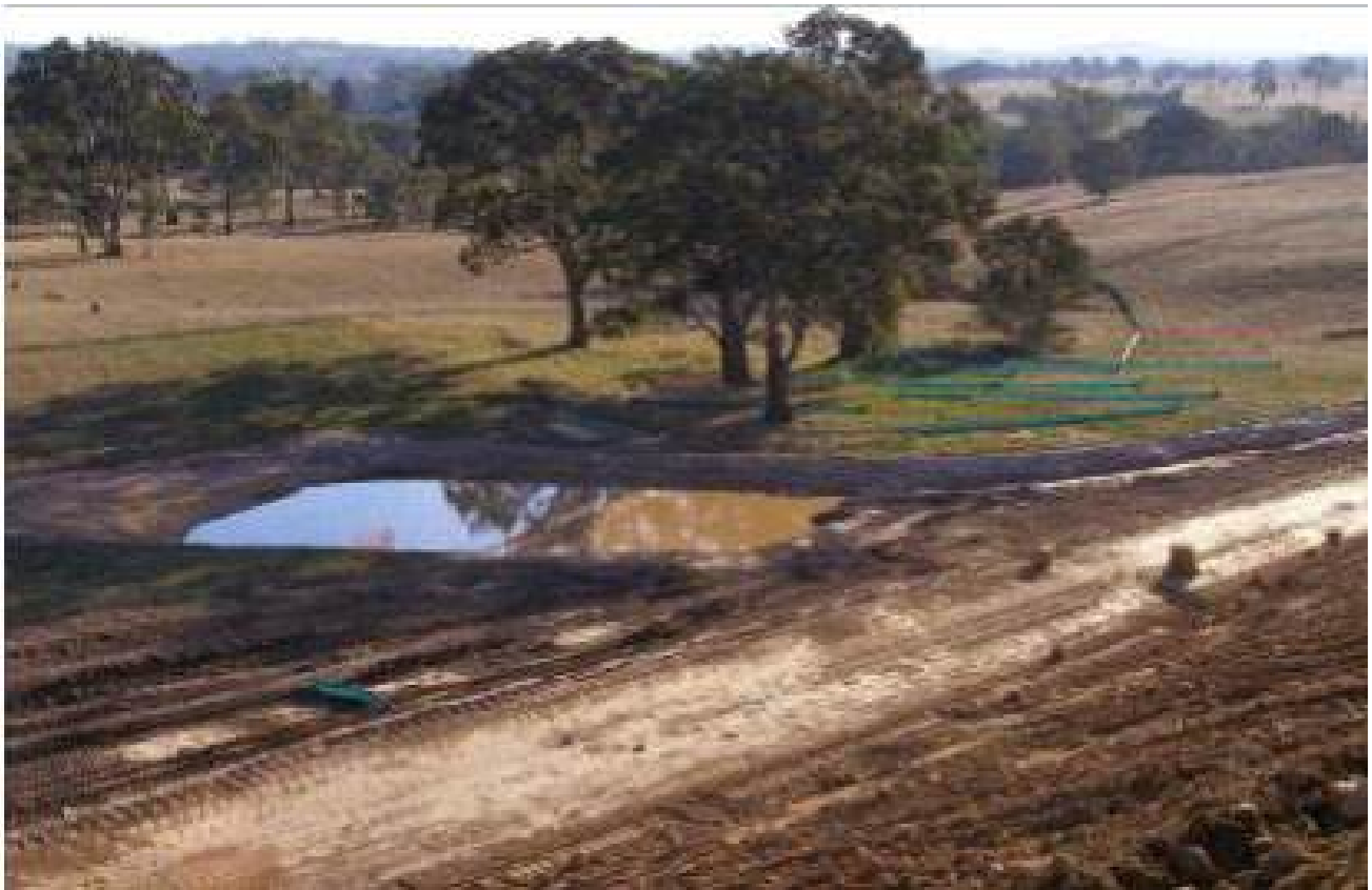
Photo 10.1 Example of construction phase sediment basin (source: VicRoads Integrated Water Management Guidelines, 2012)
