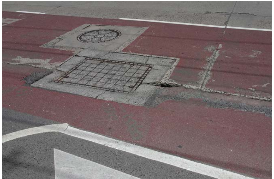
Uneven surfaces and surface breaks near utility covers can make it harder for motorcyclists to brake safely.
