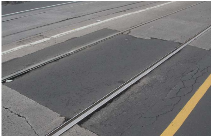
Surface cracking and breaking near tram tracks can cause motorcycle instability if they are traversed.
