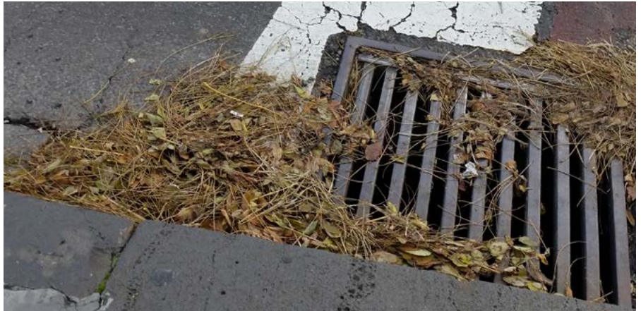
The build up of vegetation debris results in a slippery surface for motorcyclists, especially in the wet.
