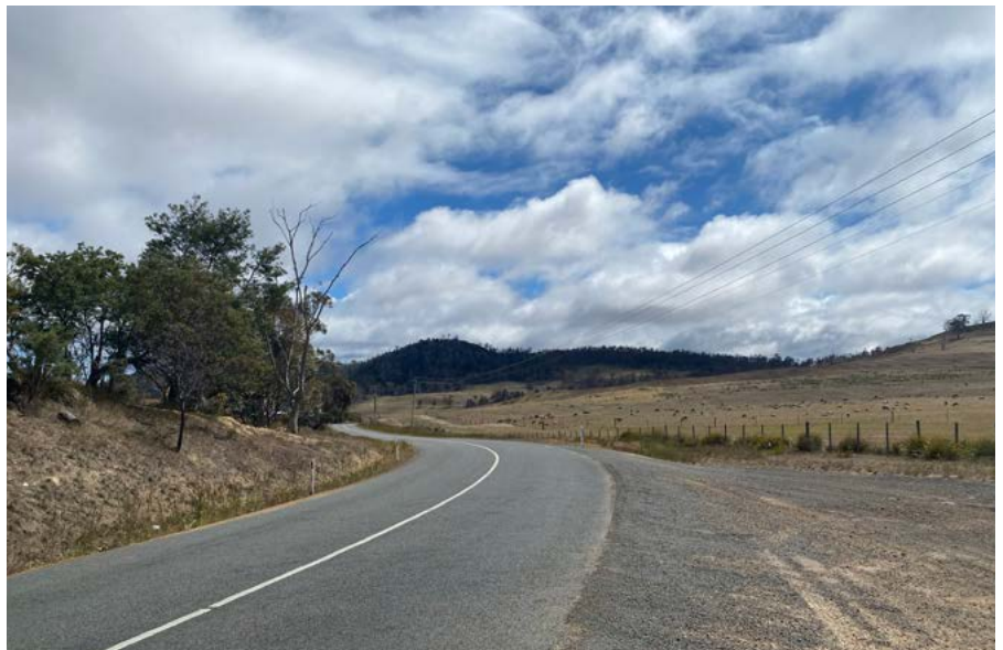
Accumulated gravel, especially when its colour is similar to that of the road surface making it indistinguishable to that of the road, is a hazard for motorcyclists.
