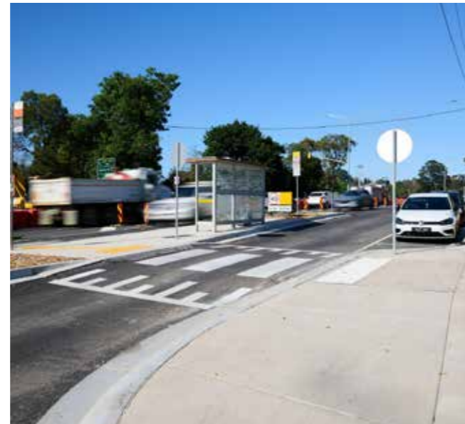
Works around the Leith Road service lane have been completed, including fresh parking for the Leith Road shops, new decorative concreting, a raised pedestrian crossing and a new bus stop.
