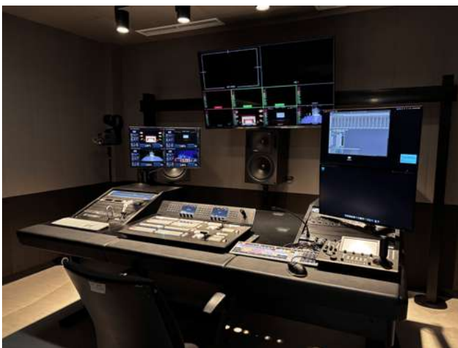
A newly installed digital media suite to support Esplanade's streaming and recording needs.
