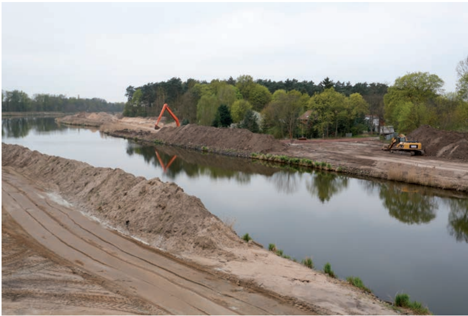
Building levees – large construction works near Fischbeck along the Elbe-Havel Canal in April 2014.
