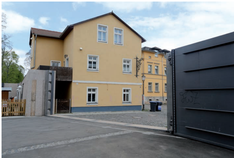
Massive flood gates and walls next to the Mulde river in Grimma.
