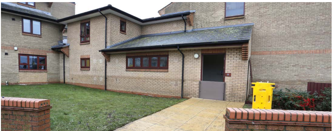
Visible water line from the surge event at a location with protection installed, including mobile defence at the door.
