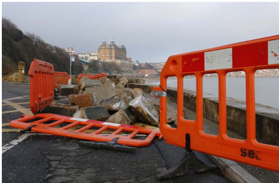
The Scarborough beach front sustained significant storm surge damage, including damage to a sea wall.
