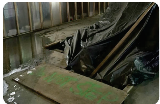
Figure 5: Example where a response cart could have prevented water from entering an escalator machinery pit (Source: Zurich Risk Engineering)
