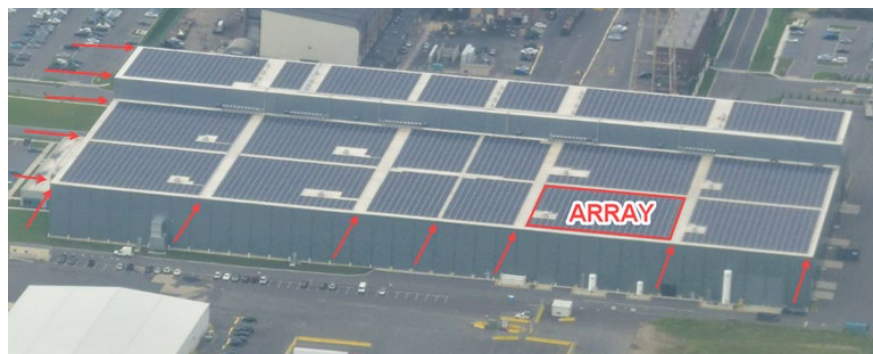
Examples of a PV array (red box) and PV system walkways (red arrows) (Source: ZRS)
