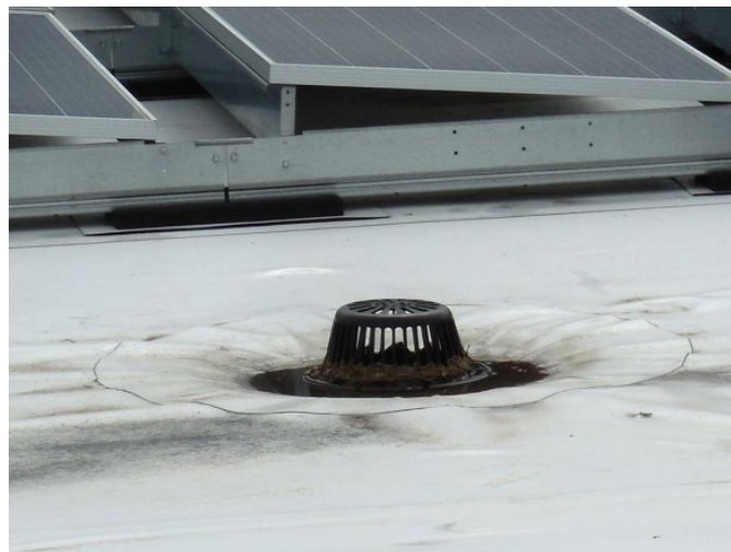
An example of a roof drain on a low-slope roof adjacent to PV modules. (Source: ZRS)
