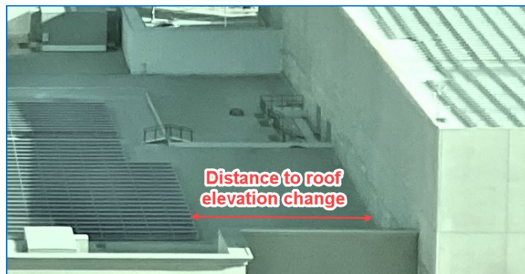
An example of a separation distance between a PV system and a roof elevation change. (Source: ZRS)
